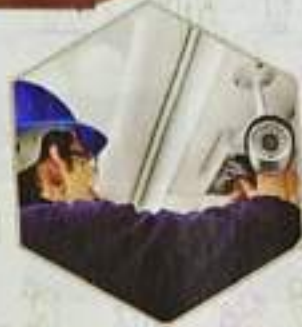
CCTV Installation (Electronics)
